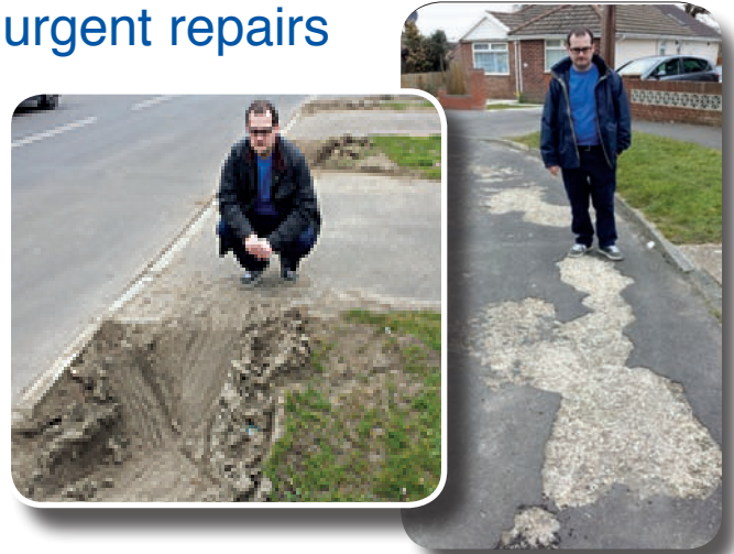
Residents pointed out wear and tear damage to the road surface and rutting of verges by inconsiderate drivers in Blackbrook Road and Southmead area. If elected, Chris will take action to remedy the situation.
