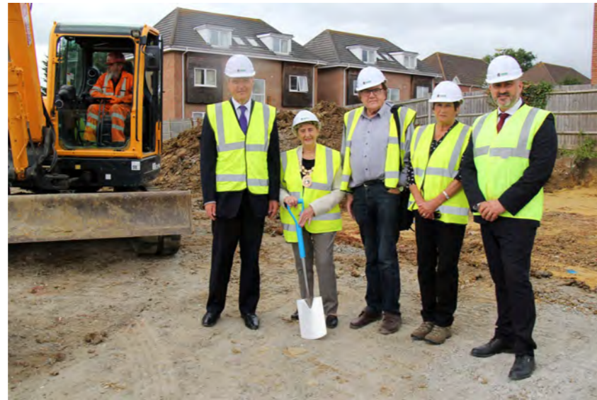
In her role as Chairman of the Housing Scrutiny Panel, Kay attended the Breaking the Turf Ceremony for the new social housing project in Highlands Road on the site of the old Hampshire Rose pub. Seen here with the Mayor, Councillor Pam Bryant and fellow councillors.
