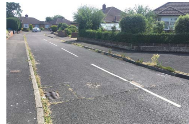
PHOTOS: Tom Davies shows where the verge by Malthouse Lane car park and gutters in the street above are weed infested.
