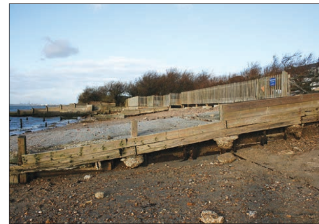
Battered by the sea: Concrete foundations (left) exposed and (above) old groynes have reappeared, almost blocking the beach.
