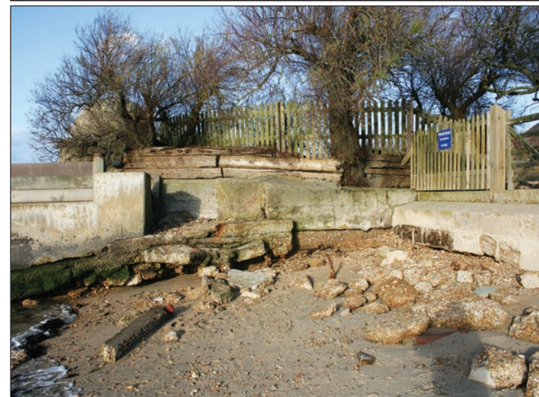
THE £1m Borough Council project to maintain and improve the sea wall at Hill Head was completed in December.
