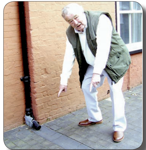
South Street resident Peter Swan emailed Geoff to say how pleased he was with new gullies installed there to prevent damp seeping into properties.
